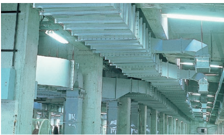
Ventilation and odor control ducts at sewage processing facilities (ET)
